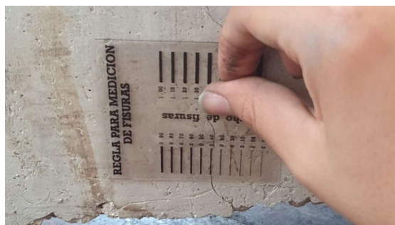
Figure 3: Crack width verification
